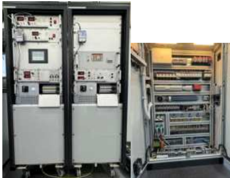
Fig. 6 New concept – Energy block and drive and pumping control switchboard
